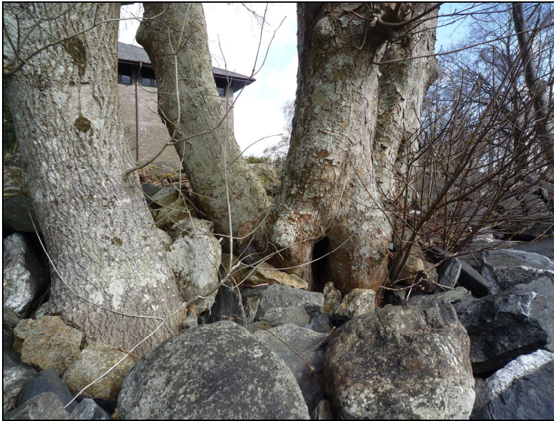
P4 – Embedded rocks/boulders and physiological disorders to base of stems in G2. Trees have limited long-term potential irrespective of proposed works
