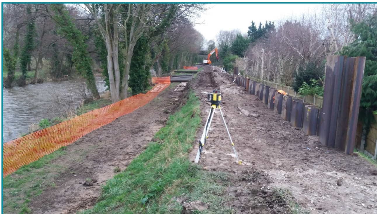
Figure 8 - several trees had to be removed along the river corridor to allow access for machinery to begin work on raising existing defences
